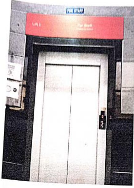
Lift no. 1 for staff
